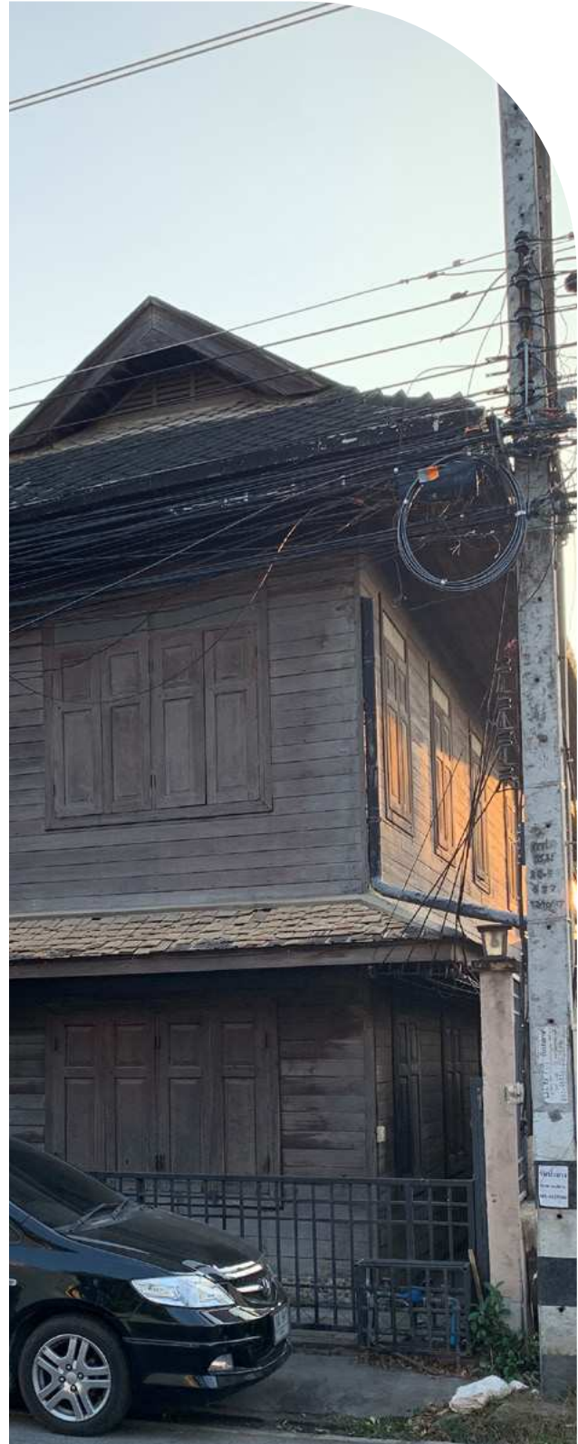
Figure 4: Electrical wiring in front of wooden house in Wat Ket Photography by: School of Public Policy, CMU, Chiang Mai, December 2019
