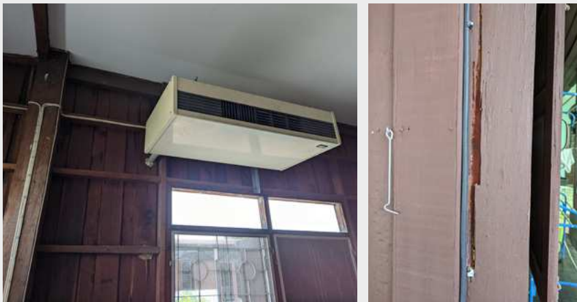
Figure 2: Hole in the ceiling in order to facilitate natural ventilation (1st); Leaking construction (2nd); Installed air conditioning system and single layer glazing (3rd); Termite damage to the construction (4th) Image Sources: Fraunhofer Institute for Building Physics IBP (Fraunhofer IBP)
