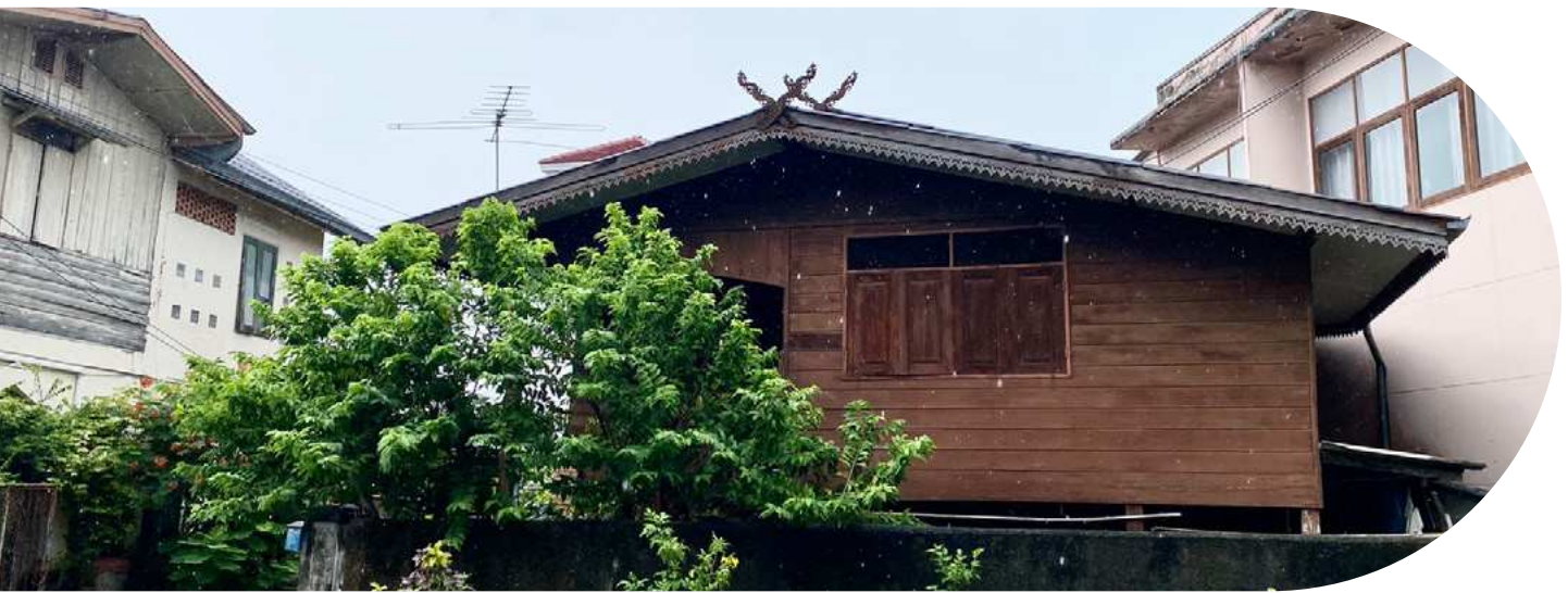
Figure 1: Wooden residential house in the Chang Moi neighborhood with kalae Photography by C. Richter, July 2022
