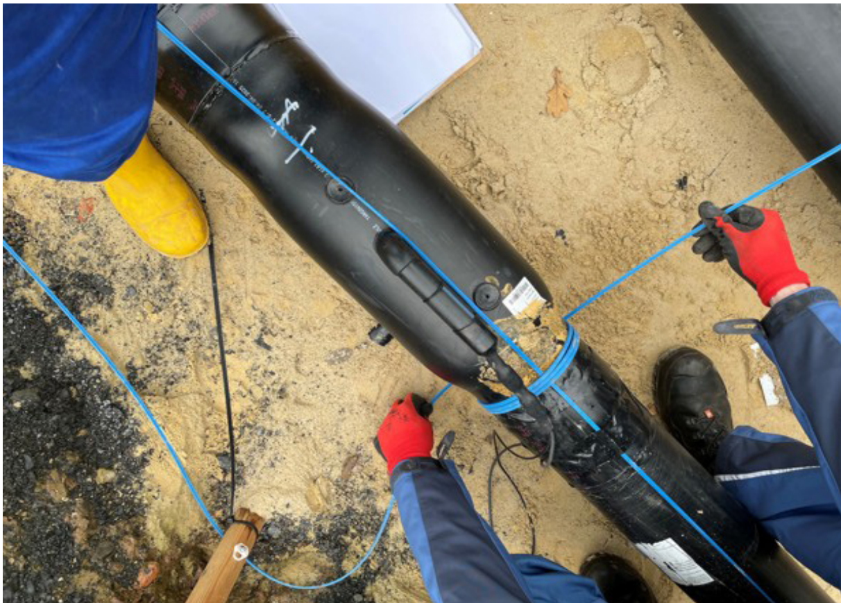
Figure 14: Joint with welded nozzle for routing the sensor cables
