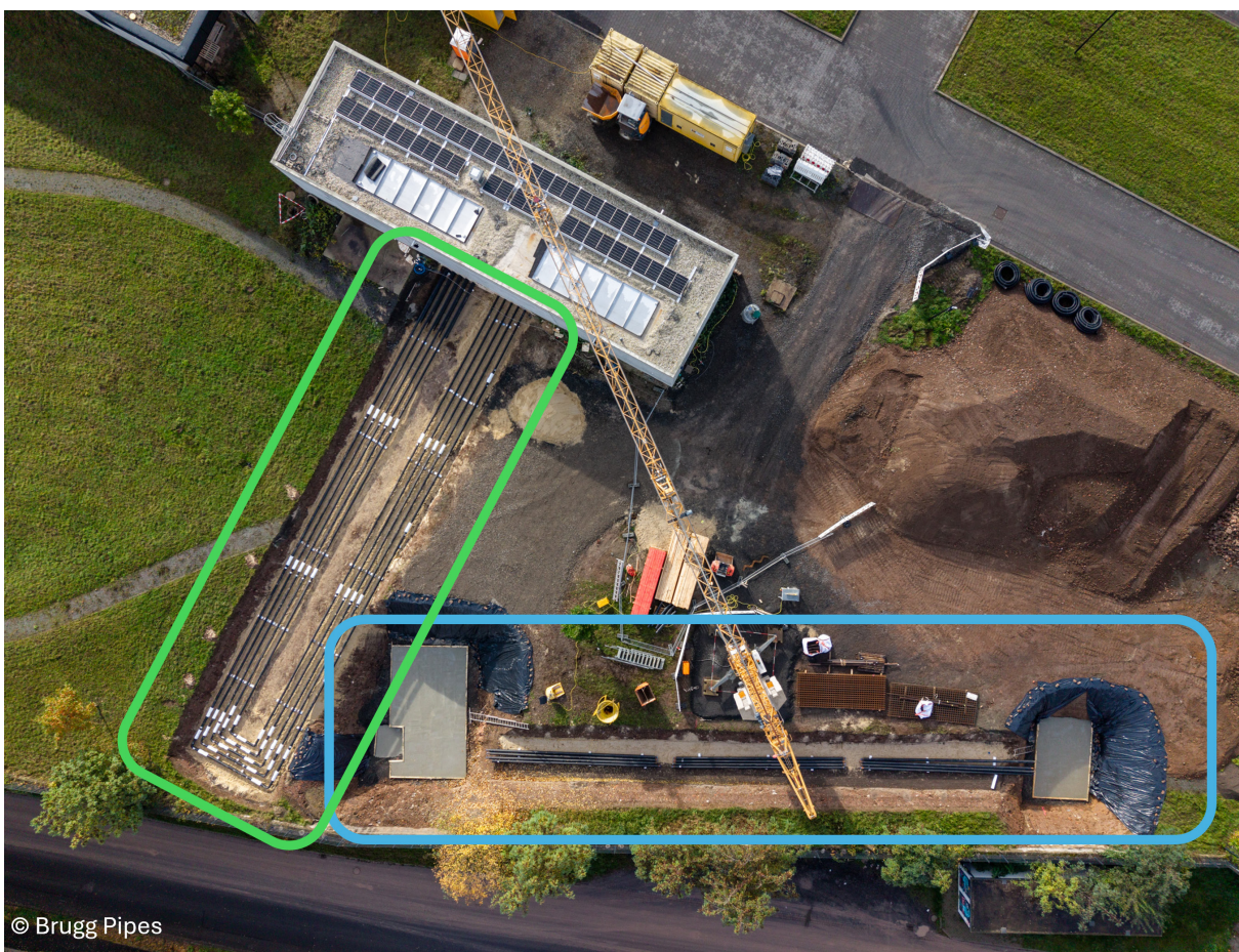
Figure 4: Aerial view of the District LAB during construction work, with the experimental fields “pipe test bench” (blue) and “flexible heating grid” (green) marked.
