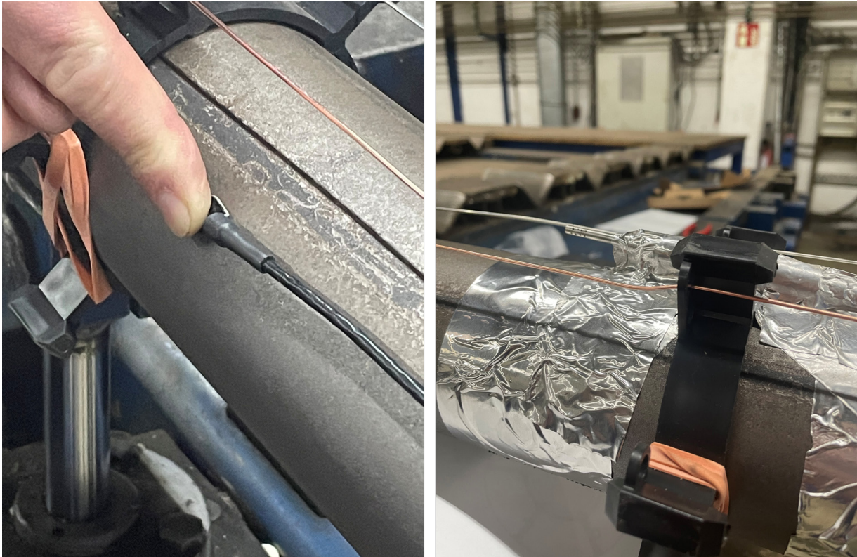
Figure 12: Installation of the humidity and temperature sensor and the surface temperature sensor in the pipe
