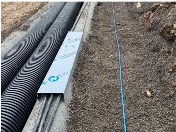
Figure 10: Extensometer - Anchor and fibre-optic cable(blue)
