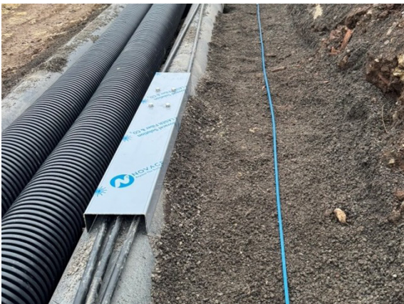
Figure 10: Extensometer - Anchor and fibre-optic cable(blue)
