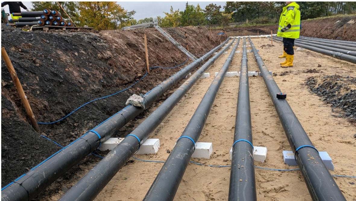
Figure 9: Installation of the fibre-optic measuring cable on the pipes by winding it around them and on the slope using wooden pegs.
