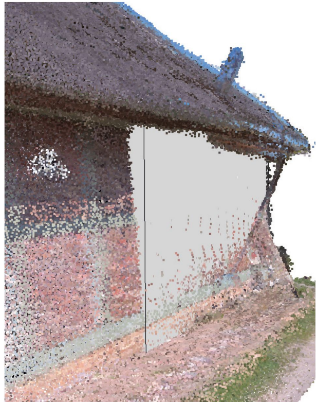
Fig. 2.4.11: Exterior wall that tilts inward
