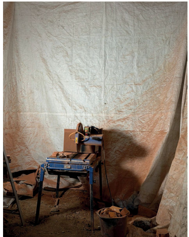
Fig. 2.3.6: Photo of areas obstructed by building materials
