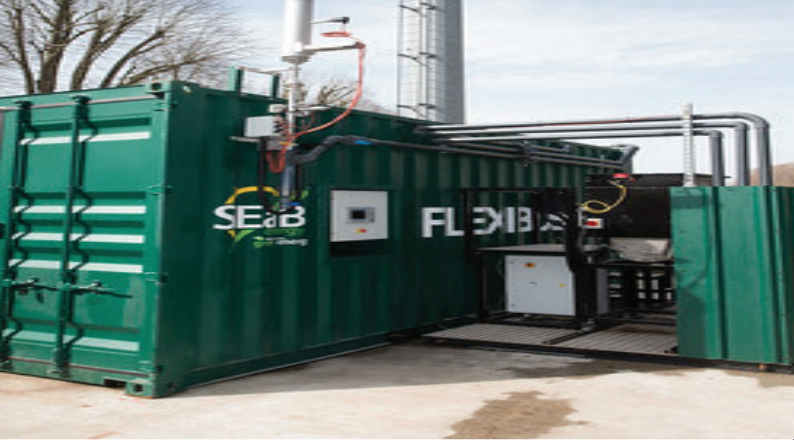
FIGURE 64- Flexibuster AD plant on site substituting waste trucks on the streets
