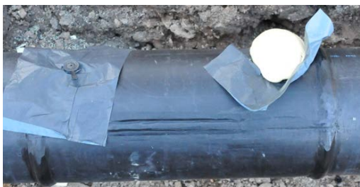
Fig. 2: Embedded extrusion sleeve section 1 after the production of the PE welds and the foaming process
