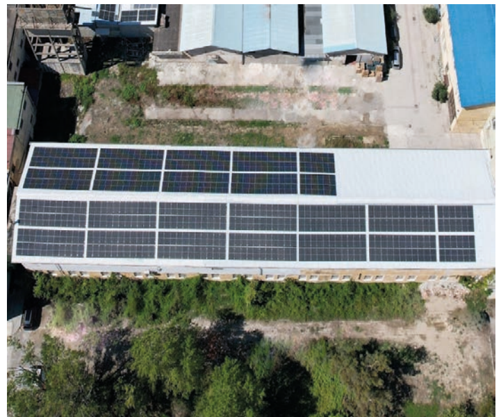
Figure 59 Use of Solar Panels to Improve Energy Efficiency
