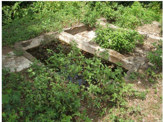
Figure 17. Old destroyed tanning pits (Own image, 2014)
