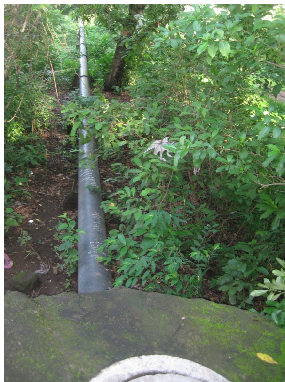
Figure 16. Wastewater collectors by the river financed by Austrian cooperation in the 90's (Own image, 2014)
