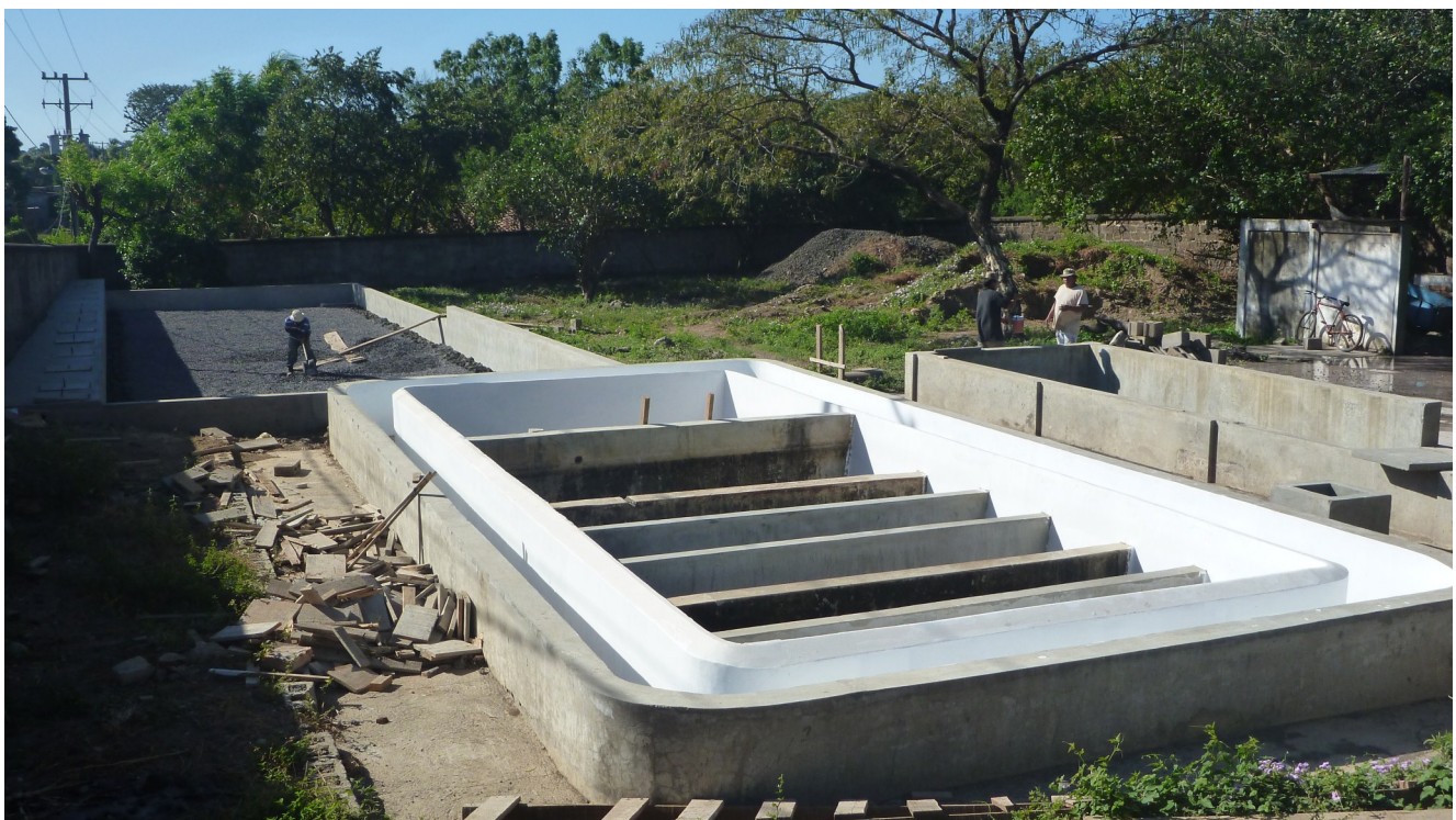
Figure 14. Pilot project, from the left horizontal filter, Filter reactor and tank for slurry (BORDA, 2013)
