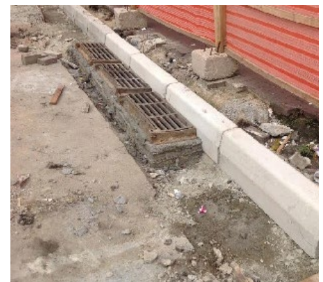
Figure 2:17 Conventional drainage (“boca de leão”) in Santo Amaro Corridor (SPObras, 2014).
