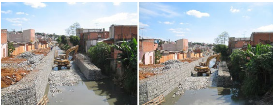
Figure 2:23 SABESP decontaminating the stream and correcting the banks with gabions (Central Leste Noticias, 2007).
