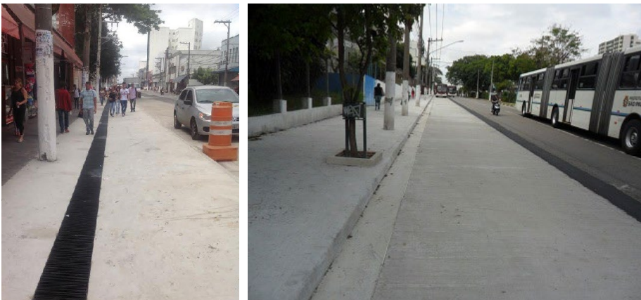
Figure 2:16 Sidewalk under construction (left) and another segment completed in Santo Amaro Corridor (SPObras, 2014).
